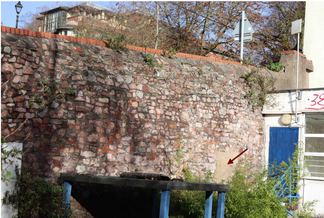
FIGURE 10: VIEW WITHIN SITE LOOKING NORTH TO RETAINING WALL AND QUEEN'S PARADE BOUNDARY WALL SHOWING (ARROWED) POTENTIAL BLOCKED OPENING INTO CELLAR SPACE BENEATH THE ROAD
